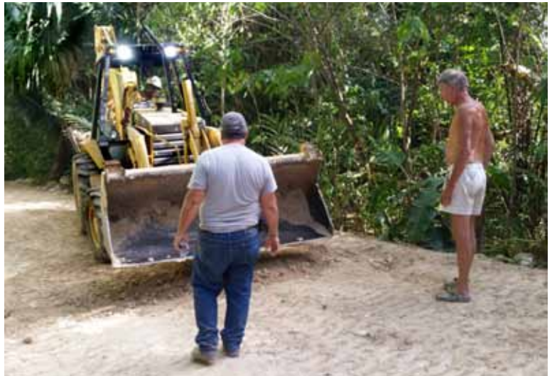
Edwardo, Max (the backhoe operator) and Bryan Weary cooperate hands-on to get the road just right.
